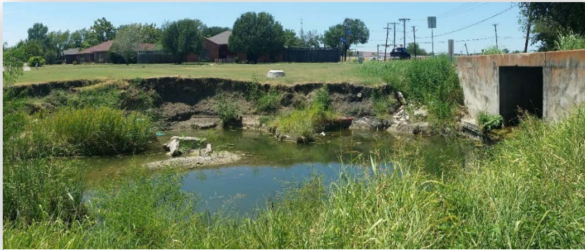
Erosion at Salmon Park
