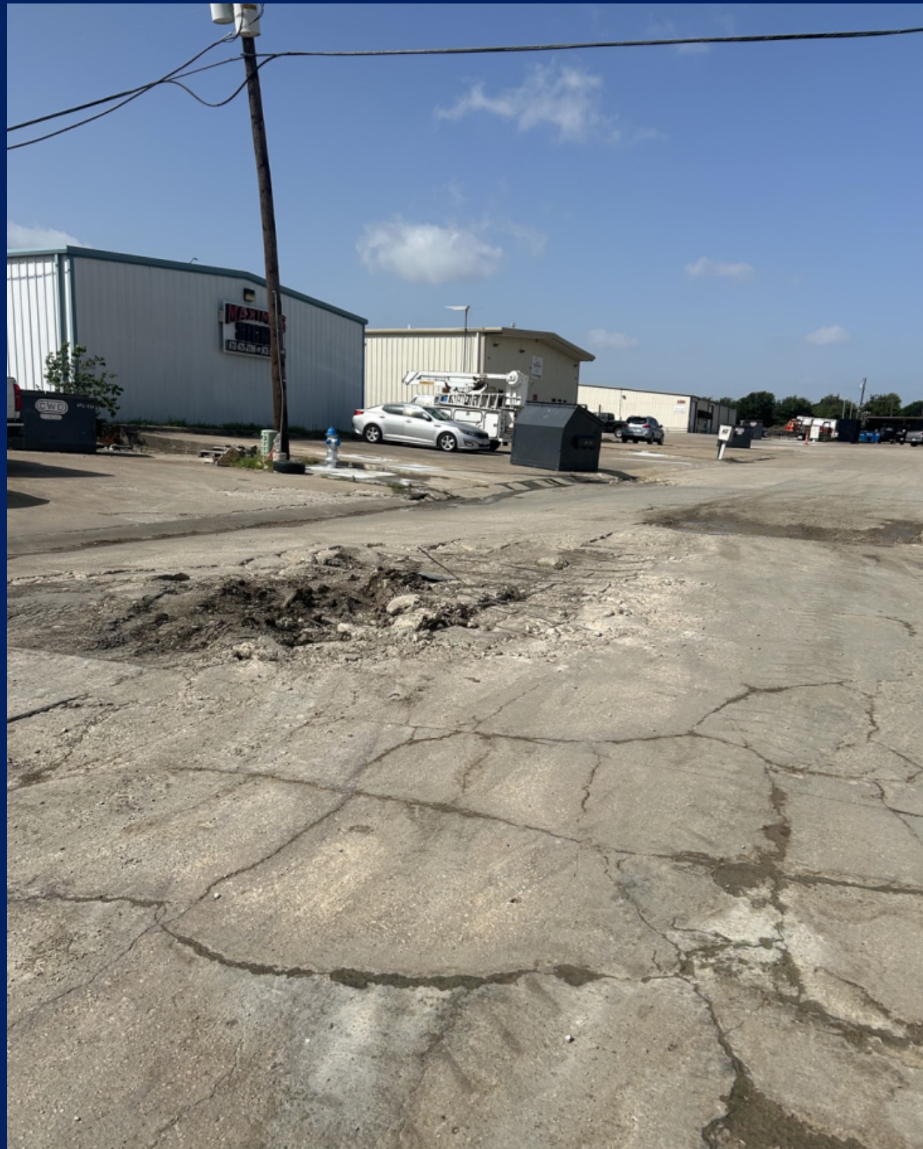
Example of PASER rating 5: Failed
