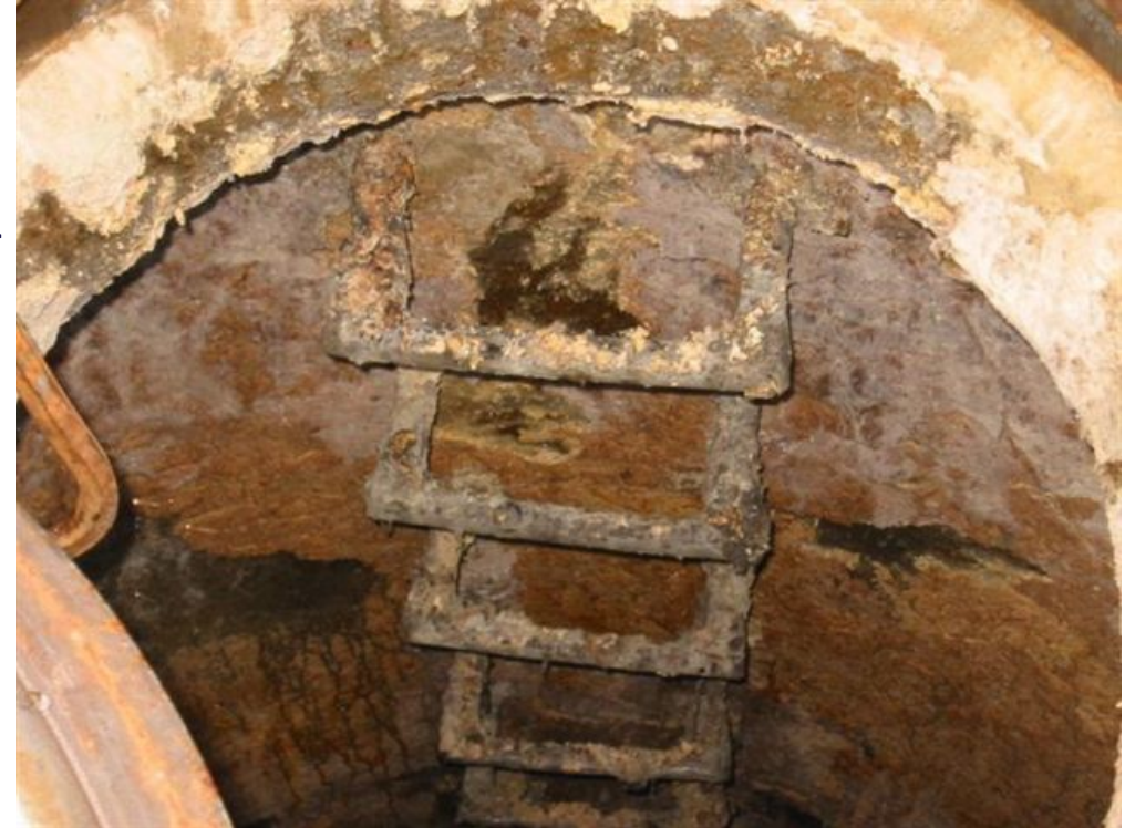
Corroded manhole due to H 2 S gas
