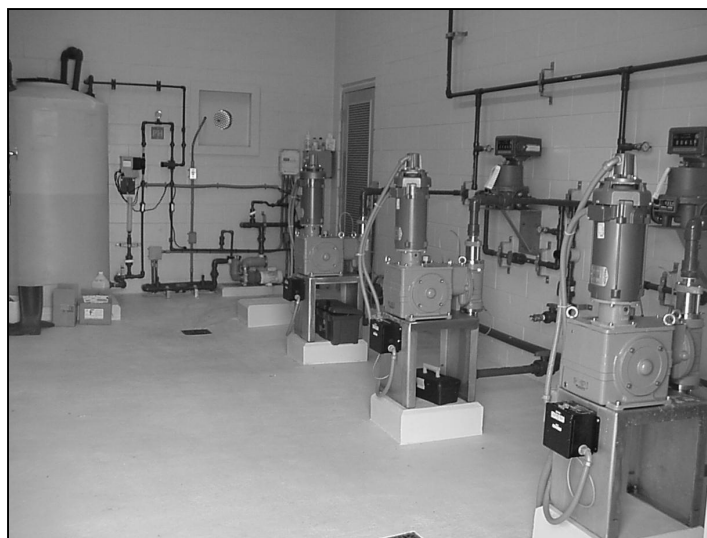
Figure 6.1 Alum Treatment System and Injection Equipment
