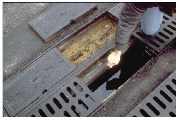
Perimeter Sand Filter
