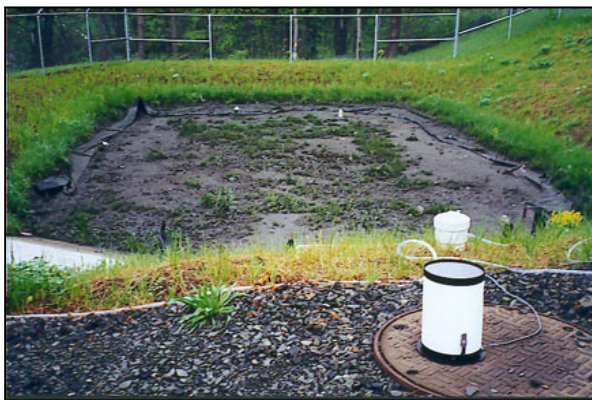
Surface Sand Filter
